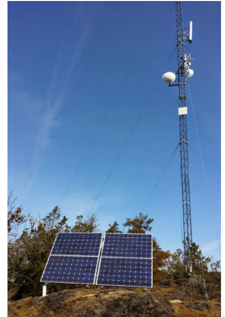
A solar powered wireless internet service provider installation
