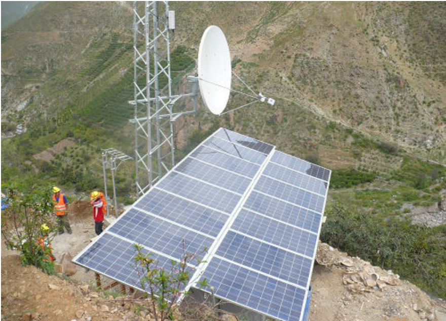
A scalable telecommunications system in Latin America
