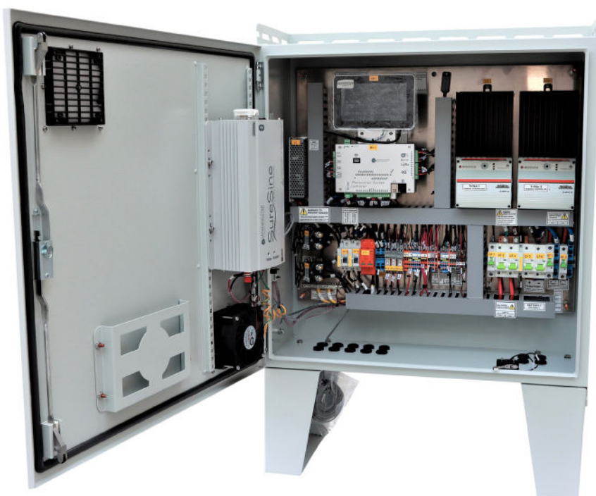
A small rural remote telecom powering system with solar charging and power conversion components on-board, in an enclosure
