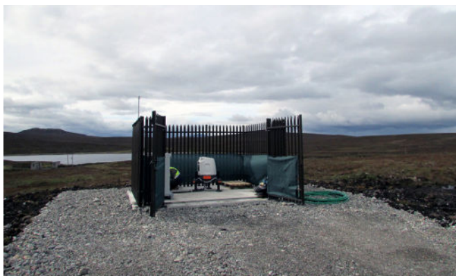
Figure 1: Permanent Wind Lidar installed with SSE
